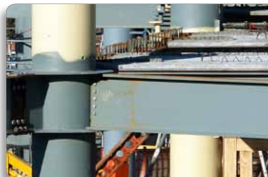
SEISMIC FORCES-RESISTING SLIDING HINGE JOINTS APPLIED AT THE UNIVERSITY OF AUCKLAND BUSINESS SCHOOL
