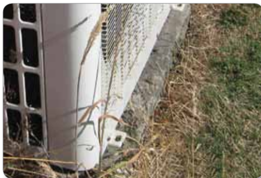
INSUFFICIENT GROUND CLEARANCE FOR HEAT PUMP OUTDOOR UNITS IS A COMMON INSTALLATION PROBLEM
