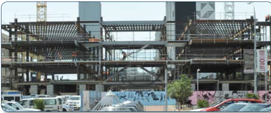
The non fire-protected, yet safe, steel-work of the cellular beams can be seen clearly in the photo of the Britomart East office building.
